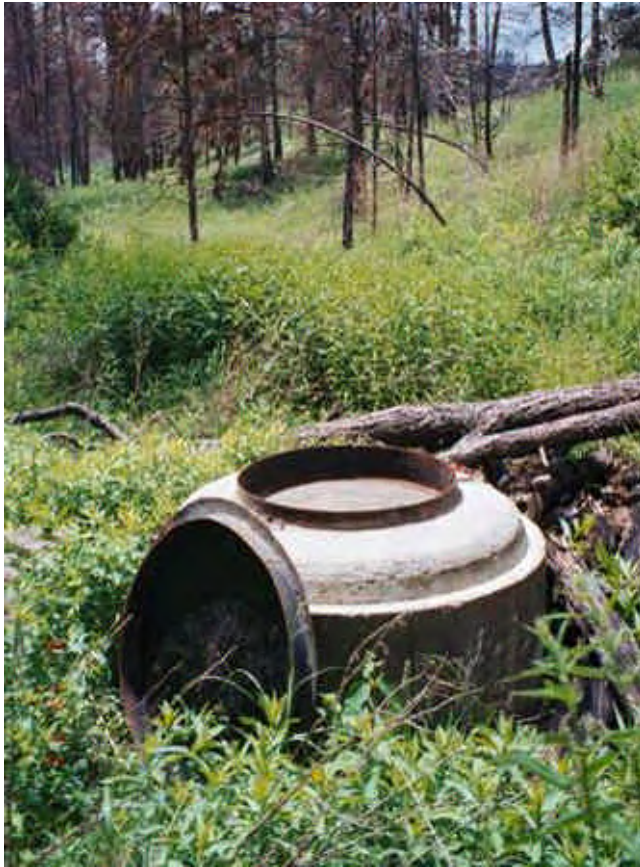
Figure 3.7: Manhole Structure at Seep/Spring near former Michaud Hotel Site (source: QE|A 2003, Roll1 AA007A)
