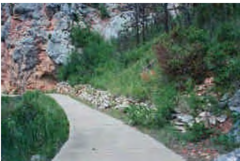
Figure 3.38: Lower trail facing north, NPS constructed stone retaining wall on right. Note impacts from vegetation and erosion. (Source: QE|A 2003, Roll5-3)
