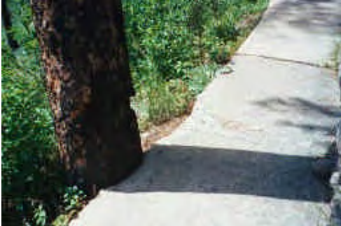
Figure 3.41: Tree at lower trail's edge about 60' north of wayside #1. Concrete is in poor condition in several areas along the lower trail. (Source: QE|A 2003, Roll5-13)
