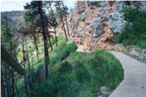
Figure 3.39: Lower trail facing north, area of CCC retaining wall to left. Cover over stones is thin in places, exposing the wall materials. (Source: QE|A 2003, Roll5-4)
