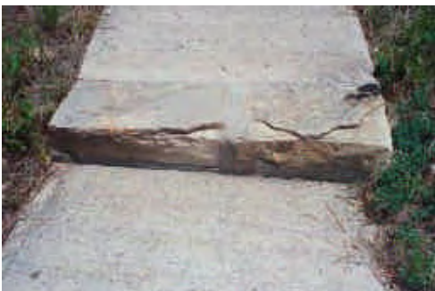
Figure 3.31: Upper trail stone step 12, cracking edge (Source: QE|A 2003, Roll4-14)
