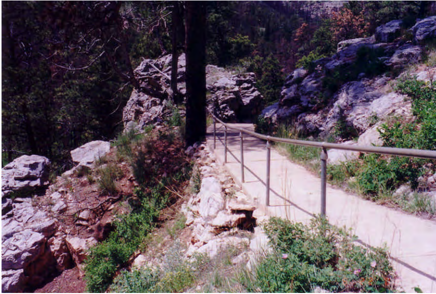
Figure 8.9: Existing conditions, Sidewalk and Railing above CCC-Constructed stone stairway (Source: QEA, June 2003)
