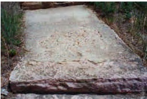
Figure 3.29: Upper trail stone step 10, deteriorating concrete (Source: QE|A 2003, Roll4-12)
