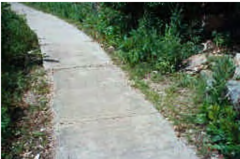
Figure 3.49: Lower trail concrete in poor condition near small cave opening located to the south of the historic cave entrance. (Source: QE|A 2003, Roll5-16)
