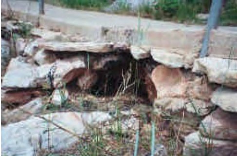
Figure 3.34: Detail of structural failure at curve in upper trail (Source: QE|A, Roll4-20)
