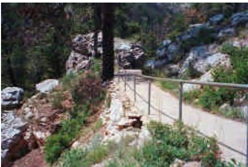
Figure 3.33: Upper trail curve near stairway, failing concrete (Source: QE|A 2003, Roll4-18)
