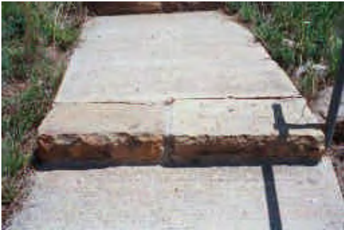
Figure 3.32: Upper trail stone step 13, pulling away from concrete (Source: QE|A 2003, Roll4-16)
