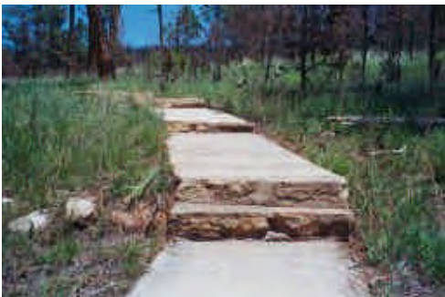
Figure 3.27: Upper trail stone steps 3, 4, and 5. The double-step configuration shown is a recent (ca. 1980s-1990s) modification and is awkward to negotiate. (Source: QE|A 2003, Roll4-9)
