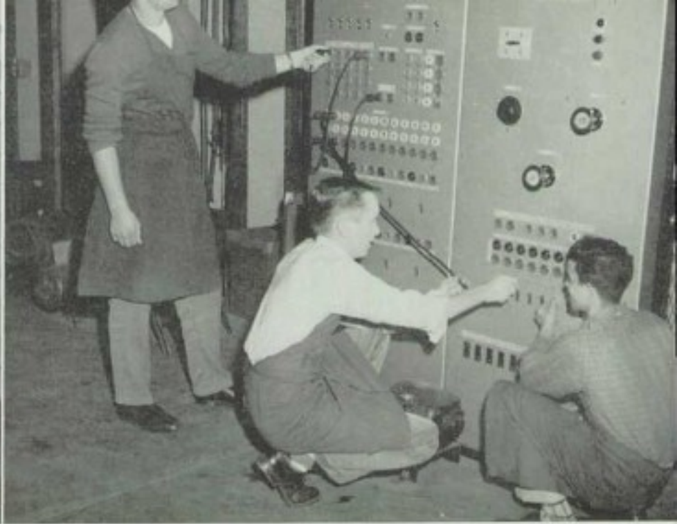
John, Norman, and Richard test the power panel in the electric shop.
